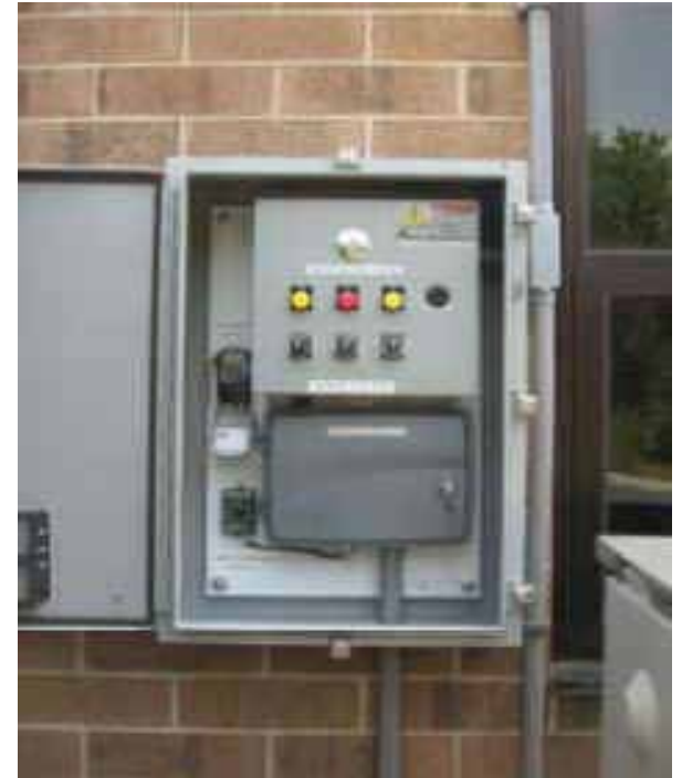
Newly installed control system at the Samuel J. Mickle School
