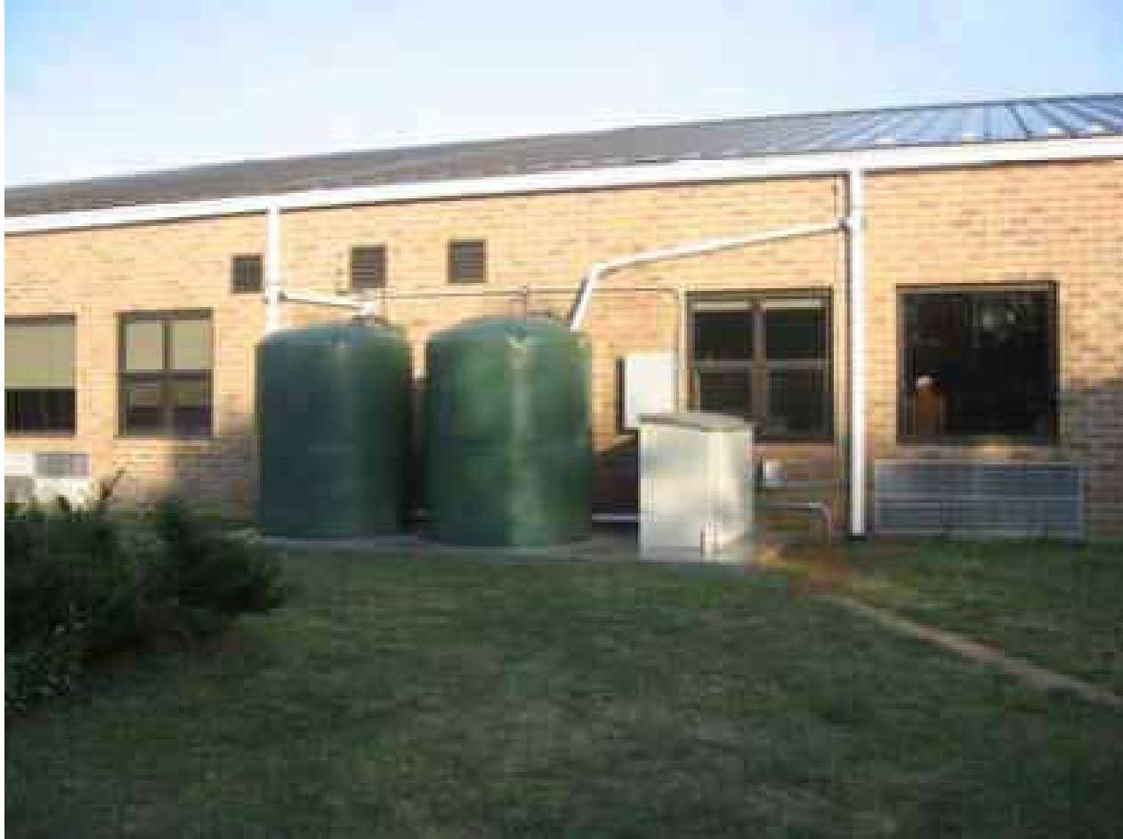
Samuel Mickle School Rainwater Harvesting System
