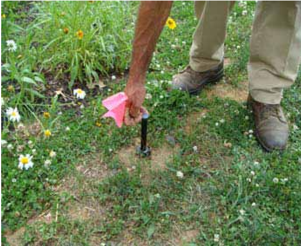
Newly installed sprinkler head at the Project WILD site at Samuel J. Mickle School.
